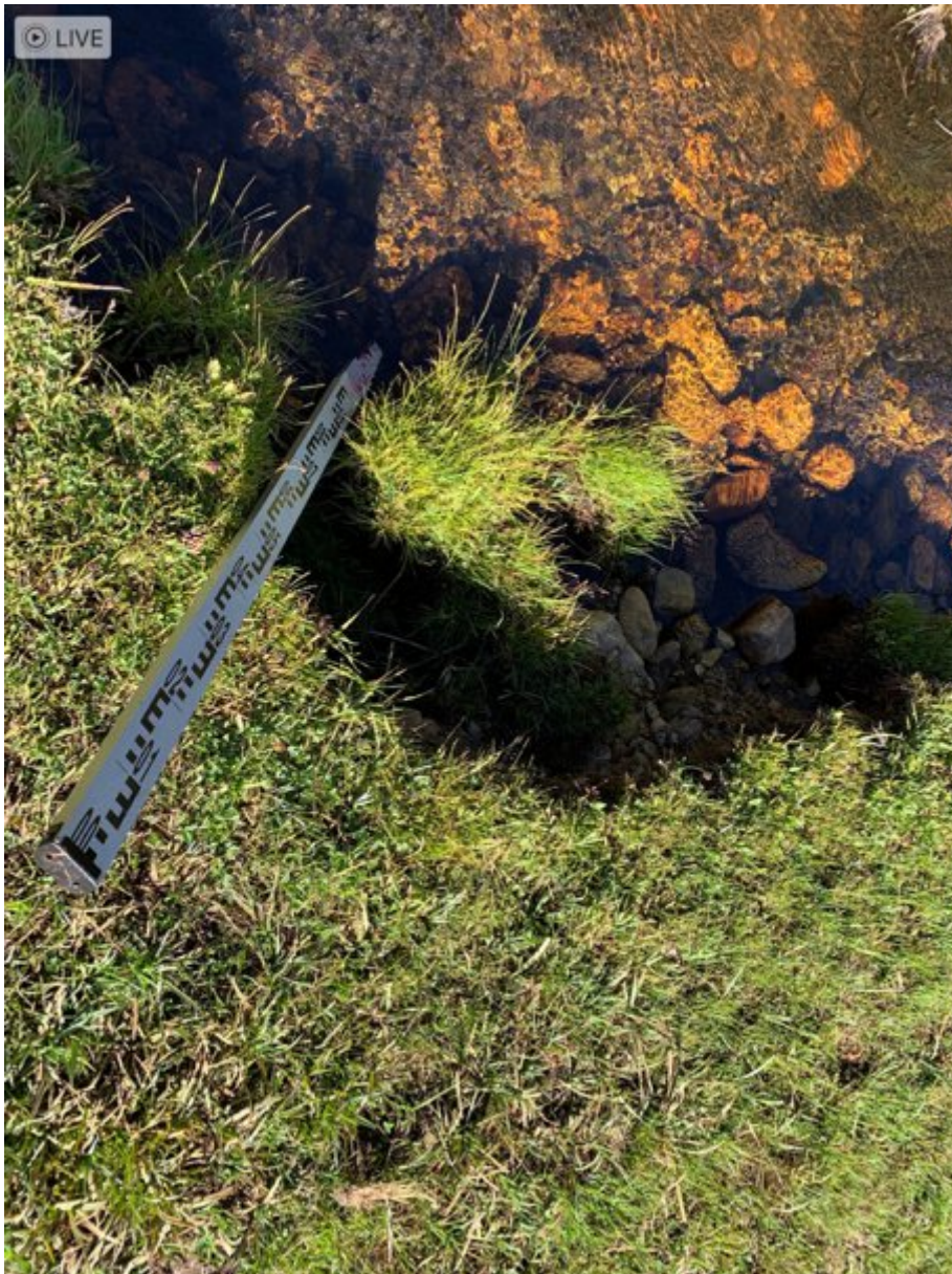
Streambank collapse. July 29, 2020.
