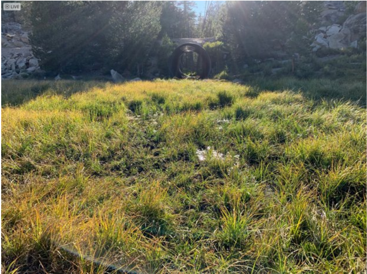
Wet sedge marsh and undercrossing pipe at Salmon Creek. Cattle appear to be grazing and trampling this area more than upstream in Big Meadow. Wildlife would normally not cause this much impact. July 27, 2020.
